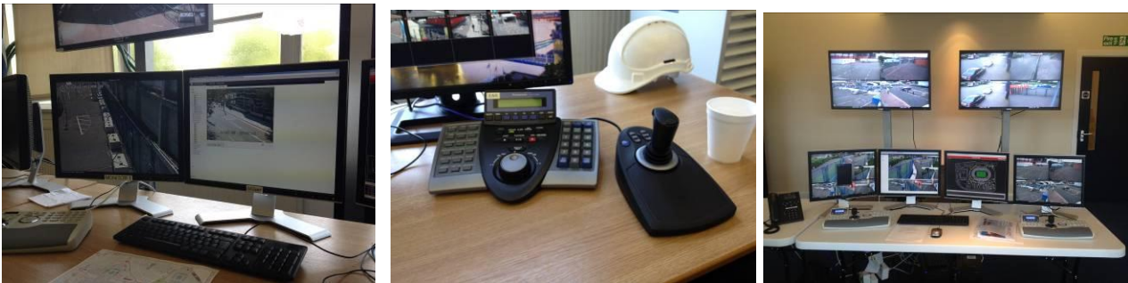
Figure 122: Where there are a number of different technologies, time to practise and 'play' with equipment will increase familiarity
