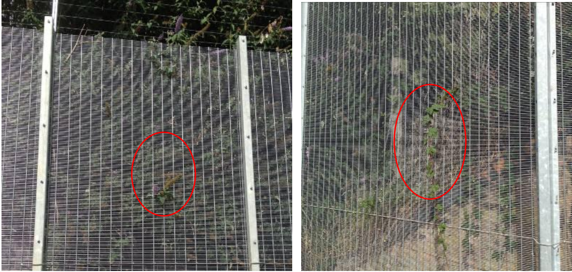
Figure 144a & b: Vegetation growing through fences (circled) triggering false alarms on the Perimeter Intruder Detection System (PIDs)
