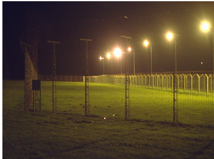
High Pressure Sodium Lighting illuminating a secure compound
