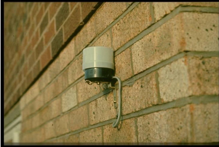
Typical photocell mounted on the wall of a building
